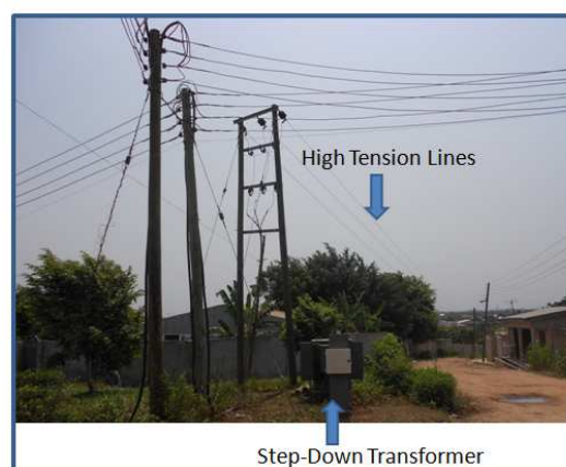
Fig1 Image of the studied building showing the high-tension power lines and the unprotected transformer
