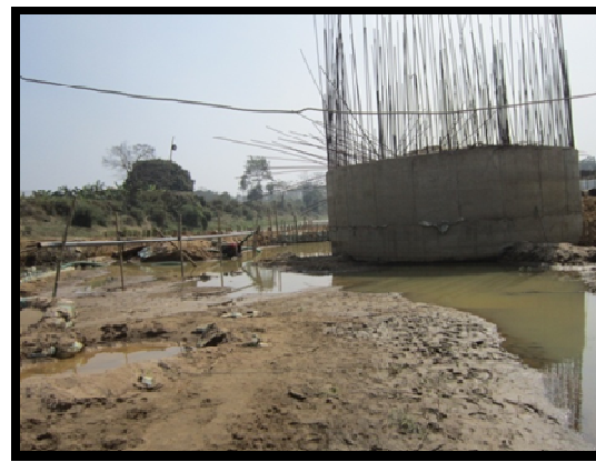
Plate 3: Construction site of Rail Bridge where the channel is blocked by an artificial road near Belonia
