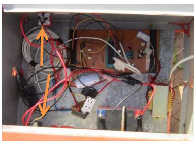
Fig 8. Electrical board, the linkage between SVM and poison-sprayer pumps
