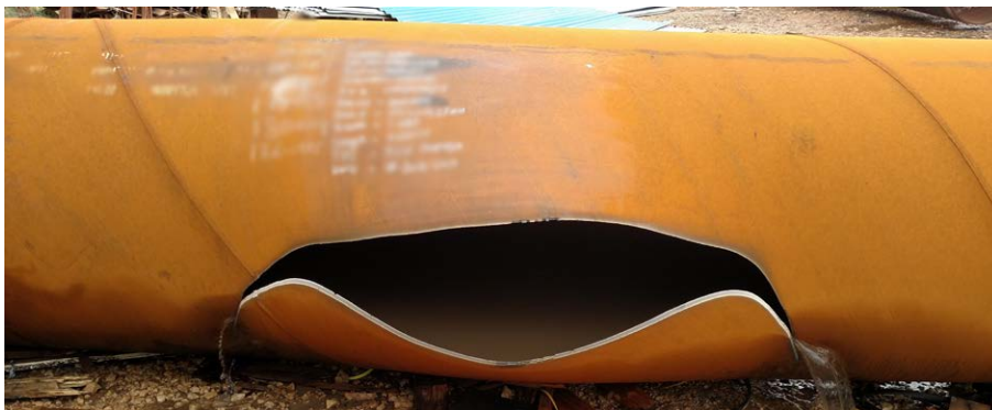
Figure 4: HSAW-1 burst pipe fracture representation, crack initiated from the pipe body and propagated through the weld bead
