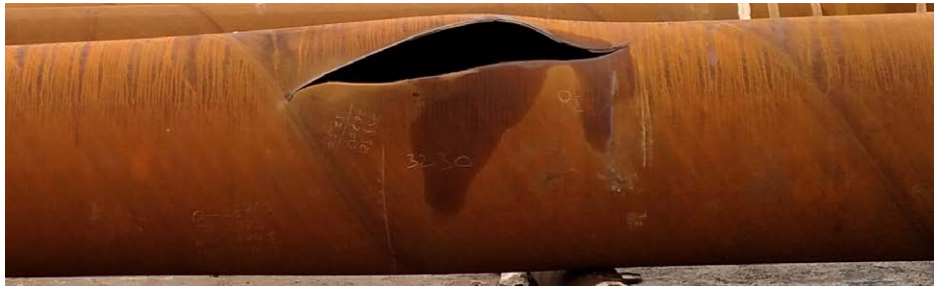
Figure 2: HSAW-2 burst pipe fracture representation, crack initiated from the pipe body, propagate but arrested by the weld bead
